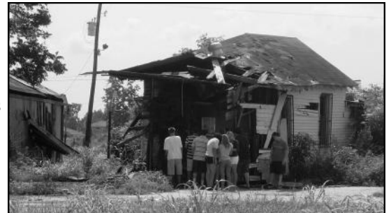
Examining a house ripped to pieces by Katrina
